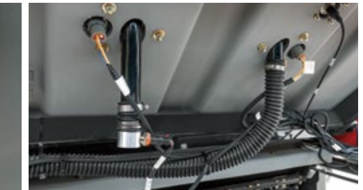
Tank pressure sensors.
